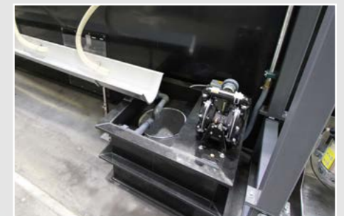
Process water collection chute with lifting station
