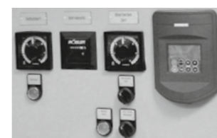
Electrical controls and compound dosing
